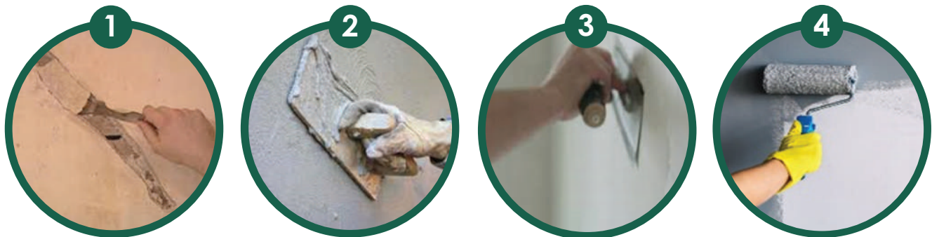
The process of cleaning, filling the cracks with plaster and painting the walls.
