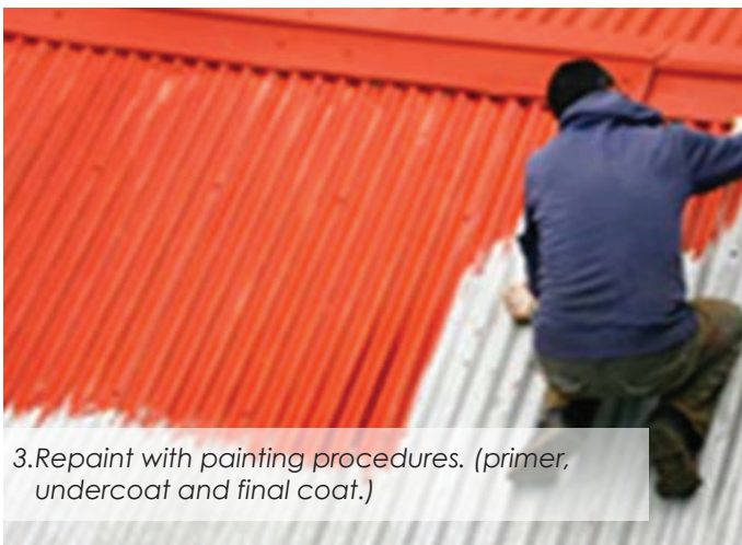
2. Apply zinc paint or rust guard on the corroded parts of the iron sheets.
