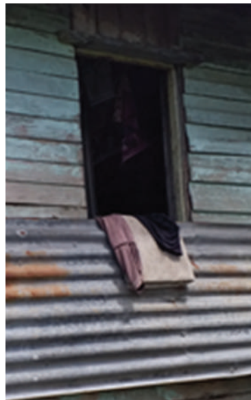
No window Covering
