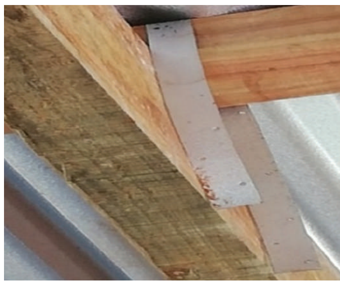
⚠ Incomplete strapping techniques
