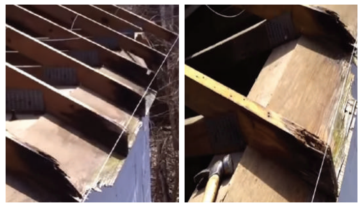
Rotten rafters due to the absence of fascia boards
