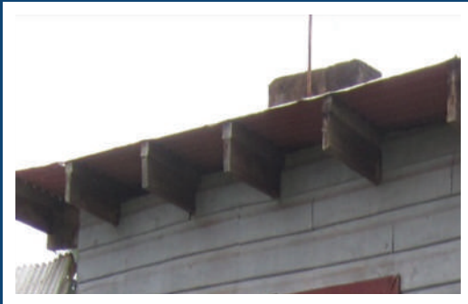
! No gutters and downpipes
