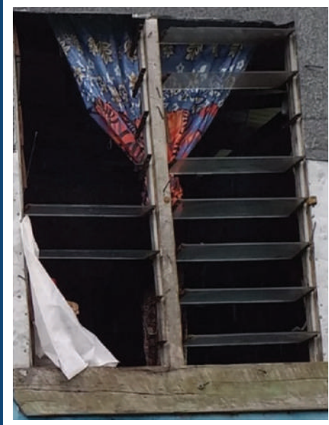
Missing Louvre blades
