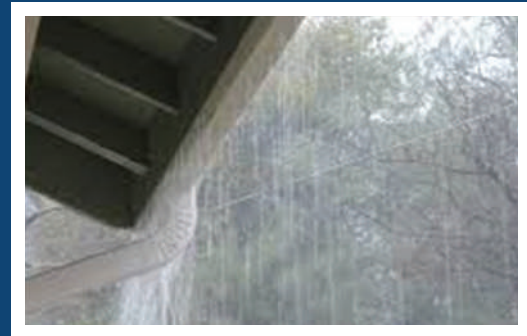
! Clogged down pipes/water overflow from the gutter
