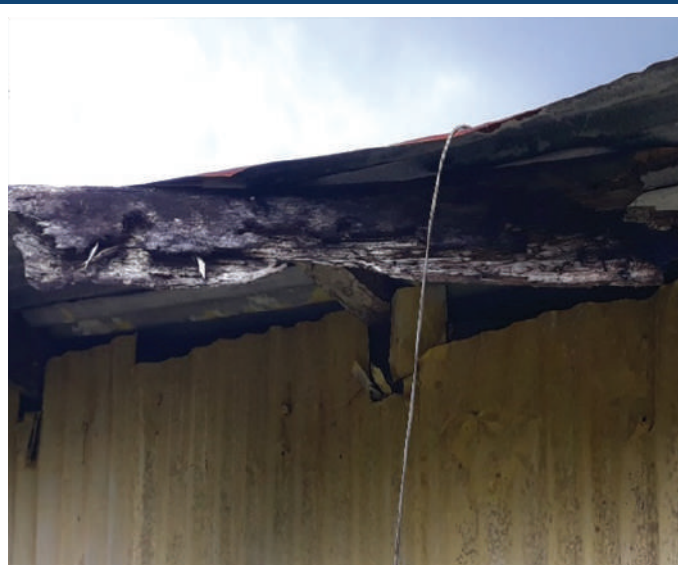
⚠ Damaged, rotten or termite infested timber
