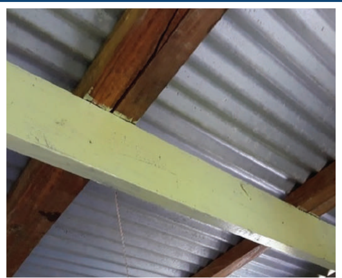
⚠ Missing or damaged fastening materials
