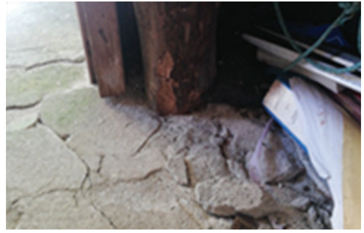
concrete floor cracks"
