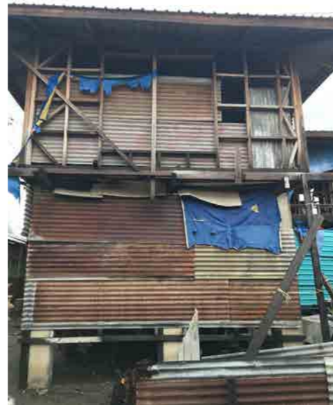
Figure 25: Incremental addition of wall finish (temporary) but structure built well. Location: Ontong Java settlement (Photo credit: John Clemo)
