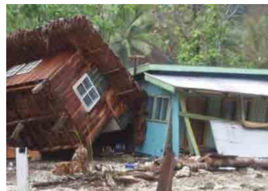
Figure 75: Without anchoring the house to the ground with footings, the entire house - no matter how well built, tied, and braced - can still tip over in a disaster event. (World Vision Solomon Islands, 2014)
