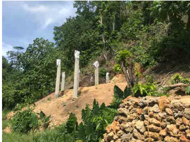
Figure 23: Only footings and posts constructed. Location: Jabros settlement (Photo credit: John Clemo)
