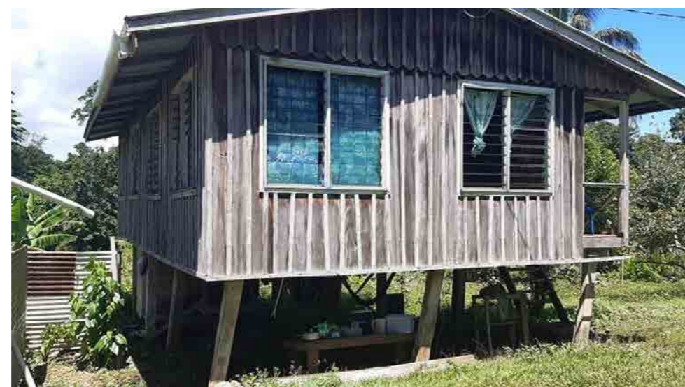
Figure 76: Structural failure of stilts due to lack of cross-bracing. (World Vision Solomon Islands, 2014)
