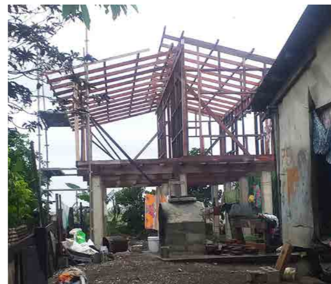
Figure 53: (Below) Hipped roof using timber for framing, galvanized steel strappings and cross bracing.
