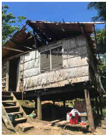
Figure 73: Roof damage due to inadequate bracing, Wind Valley settlement. (Photo credit: John Clemo)
