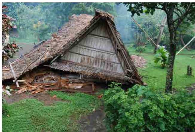
Figure 74: Complete collapse of house but relatively intact roof. (Photo credit: Kaunitz Yeung Architecture)
