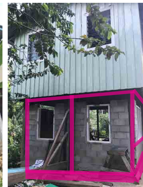
Figure 40: Photo of a house with reinforced concrete strip footing, timber posts, masonry walls and Colourbond roof. Location: Aekafo-Feraladoa settlement (Photo credit: John Clemo)
