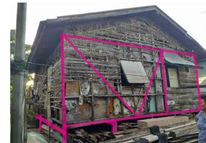
Figure 17: Photo of a house which withstood Cyclone Namu (1986) with 'copper' roof added since. Location: Fishing Village settlement (Photo credit: John Clemo)
