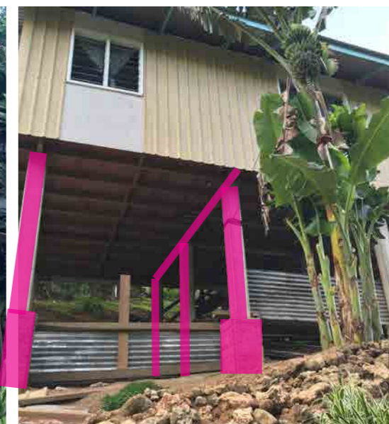
Figure 39: Photo of a house with reinforced concrete stepped footing and reinforced concrete column. Location: Aekafo-Feraladoa settlement (Photo credit: John Clemo)
