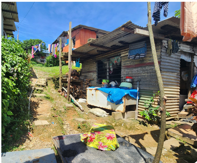
Figure 12 – Poor electricity and water connection
