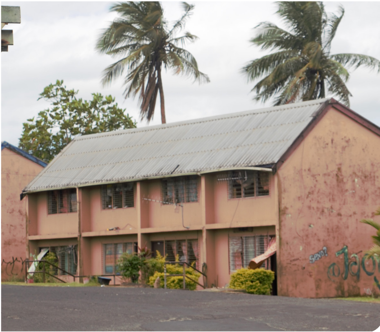
Figure 8 - Guttering on a Barrack Unit in a PRB Estate in the Nasinu area that needs to undergo maintenance work.
