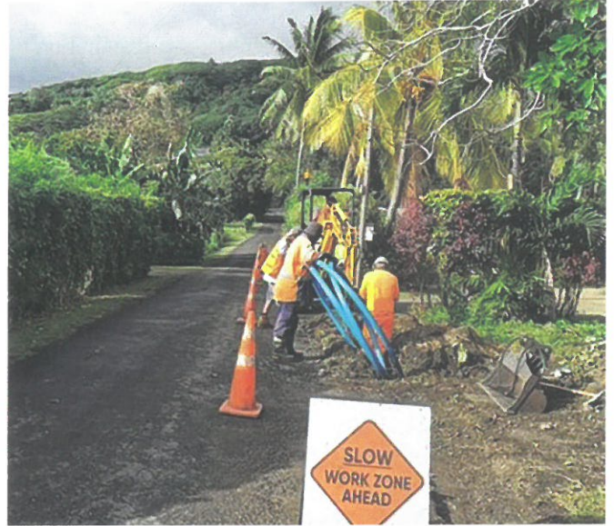
Upgrading work underway at the Tupapa area, Cook Islands, where a corroded galvanised pipeline was replaced with a new PE (plastic) pipeline that will last up to 100 years. Photo: TTV
